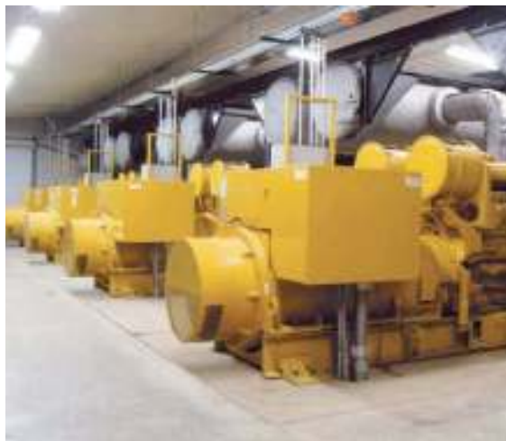
Rock Falls Electric owns seven 1,825-kW diesel generators. Five of the units are standby generators for Illinois Municipal Electric Agency.
