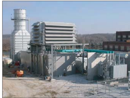
Empire District Electric Company Riverton, Kansas
