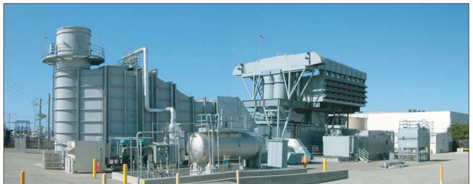
Miramar Energy Facility, San Diego, California
