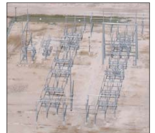
KCP&L South Harper Substation Peculiar, Missouri
