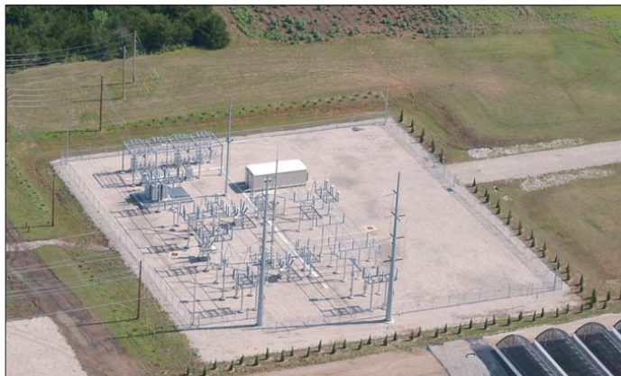
Ottawa Southeast Substation, Ottawa, Kansas
