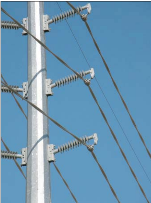
ADM Beaver Channel Transmission Line, Clinton, Iowa
