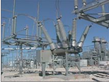
City Utilities of Springfield Springfield, Missouri
